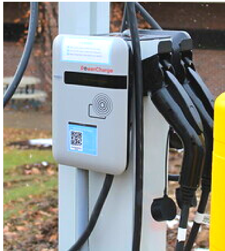
NEW EV CHARGING STATIONS AT PCC
